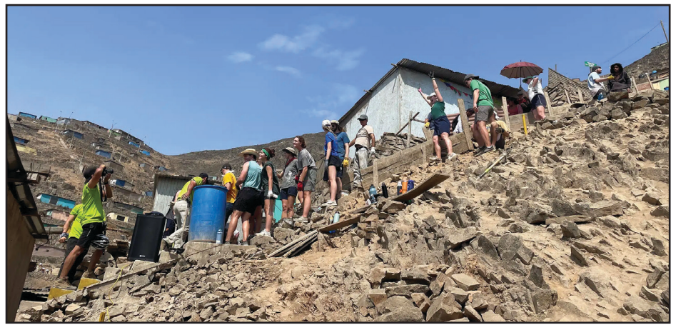
Amanda, Pitt students, and other missionaries help build stairs outside Lima, Peru.
